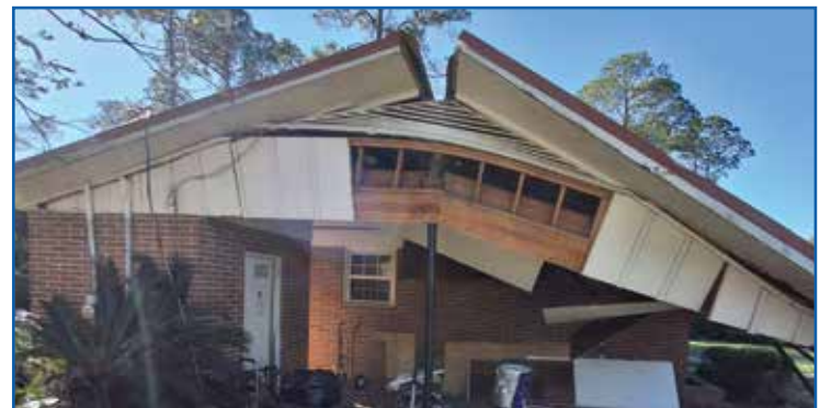
The hurricanes that devastated much of the Southeast destroyed this house in Valdosta, Ga. Photo from Colin Monk.
