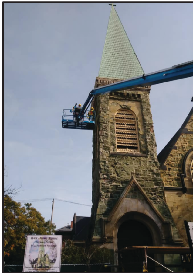
Greenstone UMC in Chicago's historic Pullman District is receiving a facelift including a new roof and stabilization of the bell tower.
