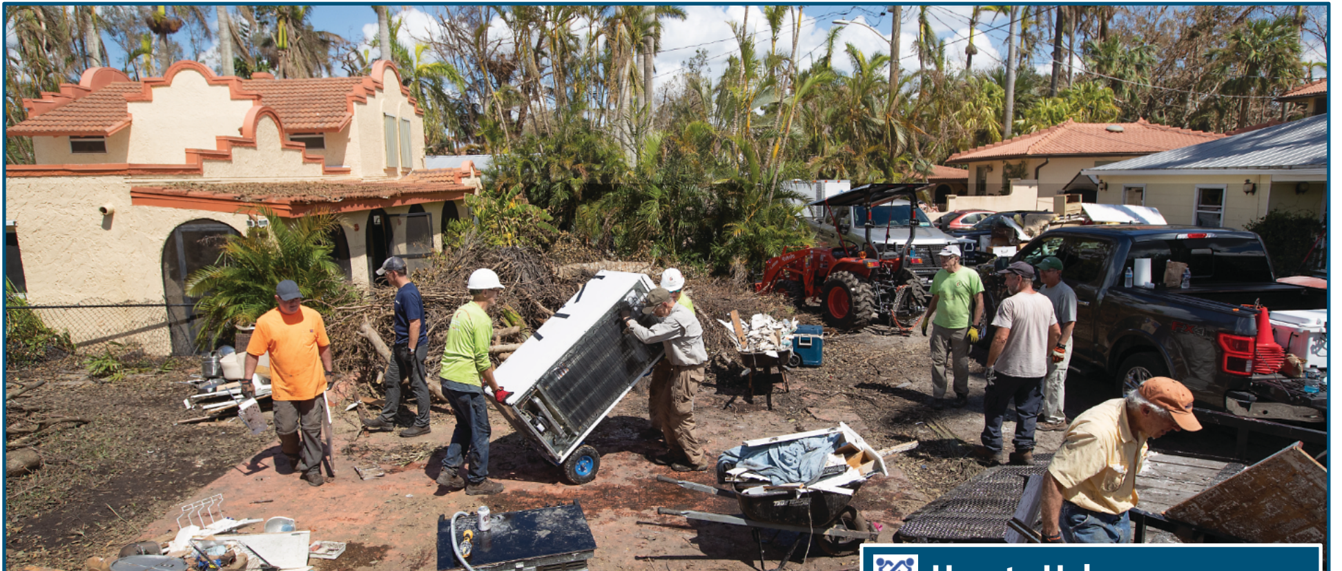
Members of a volunteer team from the North Georgia Conference of The United Methodist Church clean out a home in Fort Myers, Fla., that was flooded by Hurricane Ian. Photo by Mike DuBose, UM News.
