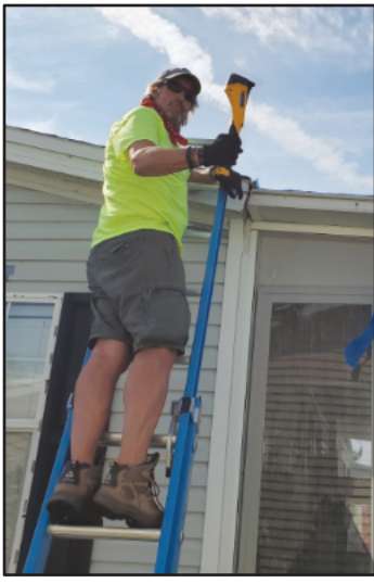
Jack Wilson from the Michigan Conference helps repair a roof damaged by Hurricane Ian in Florida.
