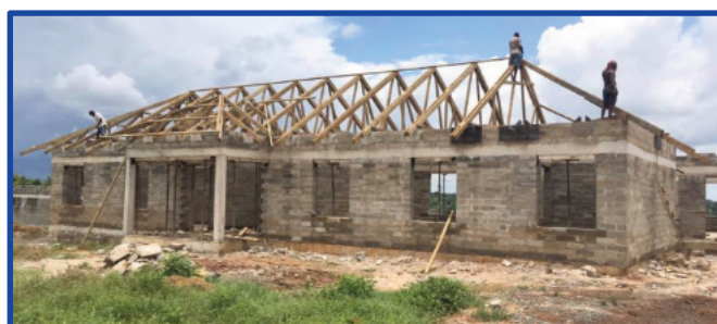
Construction crews work on installing the roof on the Global Mission Secondary School in March.
