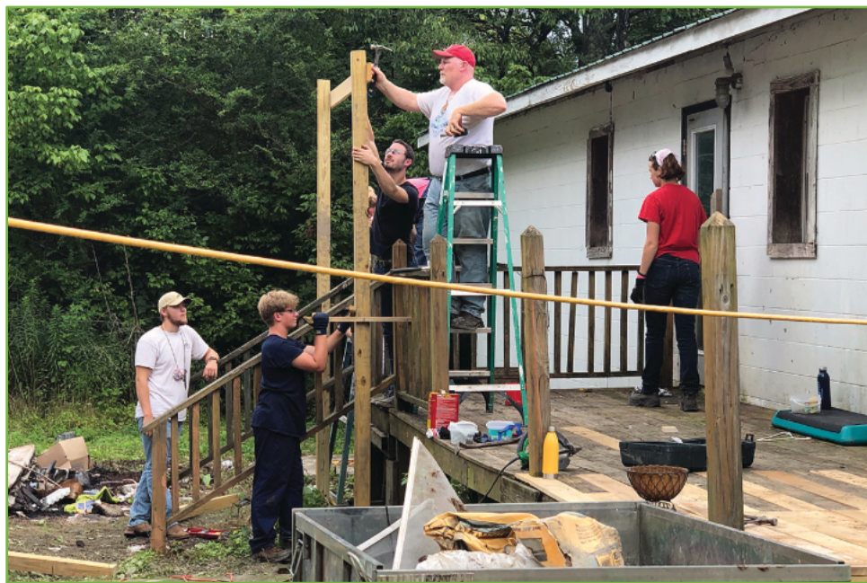
Youth and adults from Oregon United Methodist Church and St. Mary's Catholic Church, both in Oregon, Ill., repair the porch on a home in Tracy City, Tenn. The team volunteered with Mountain T.O.P., a ministry that serves families in the Cumberland Mountain region of southeast Tennessee. Photo by the Rev. Thomas Kim, UM News.
