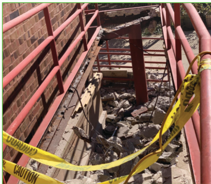
A rusty ramp originally built in 1979 is being replaced as part of the church's renovation project.
