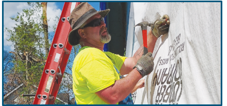
Randy Miller helps repair the outer shell of a damaged home in Rolling Fork, Miss.
