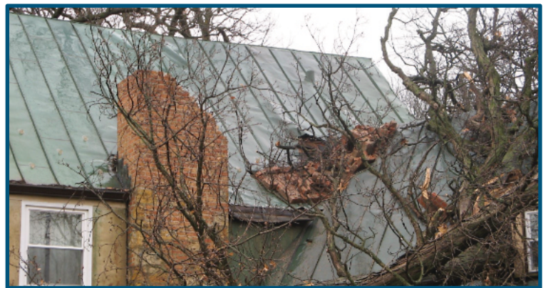
The manor house at Camp Reynoldswood, Dixon, suffered roof damage from an April 4 tornado.
