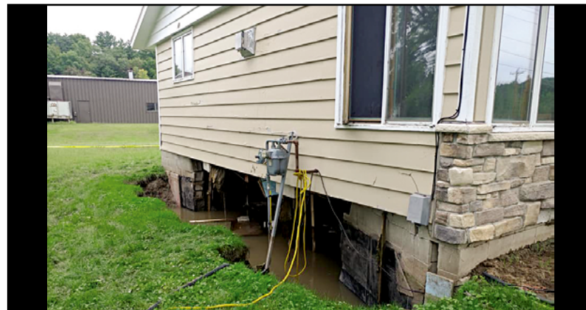
Flood waters leave extensive foundation damage to several homes in Elroy, Wisconsin.
