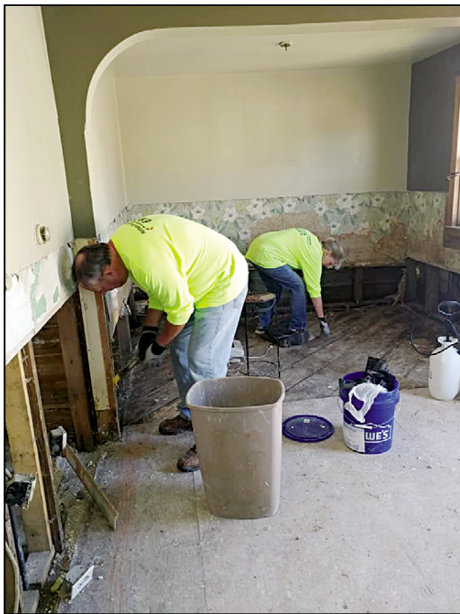
Volunteers work on mold remediation inside several homes by removing flood soaked walls and insulation.
